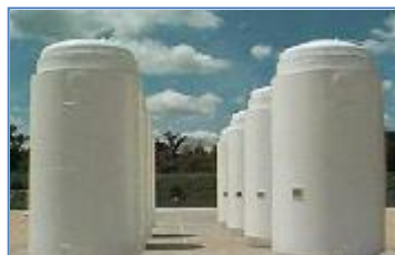
3 On Site Fuel Storage
